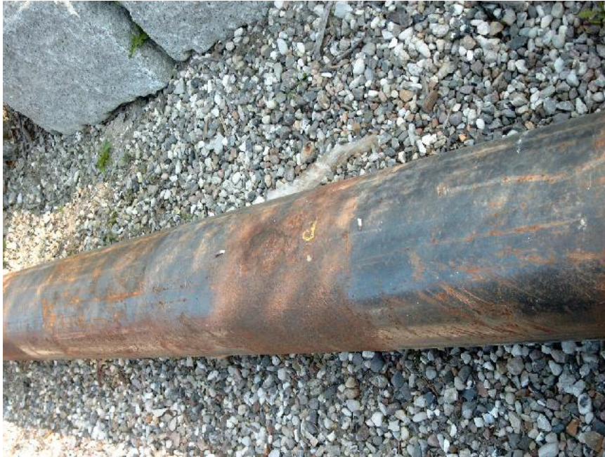
Fig. 2. Corroded 6" test pipe. Corrosion pitting is up to 5-6 mm. Insulation removed to portray the corrosion pitting. Pitting is left to the "P" mark (upside down) in the middle.
